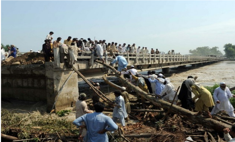
Figure 02: Extreme scour at bridge abutment of Sardaryab Bridge on river Kabul during flood, 2010
